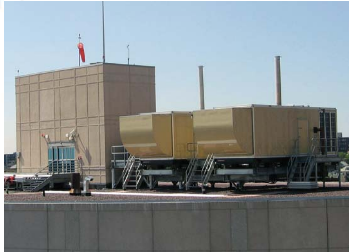
Figure 3: Locating generators on rooftops can aid exhaust re-entrainment design considerations but can complicate vibration and noise control.
