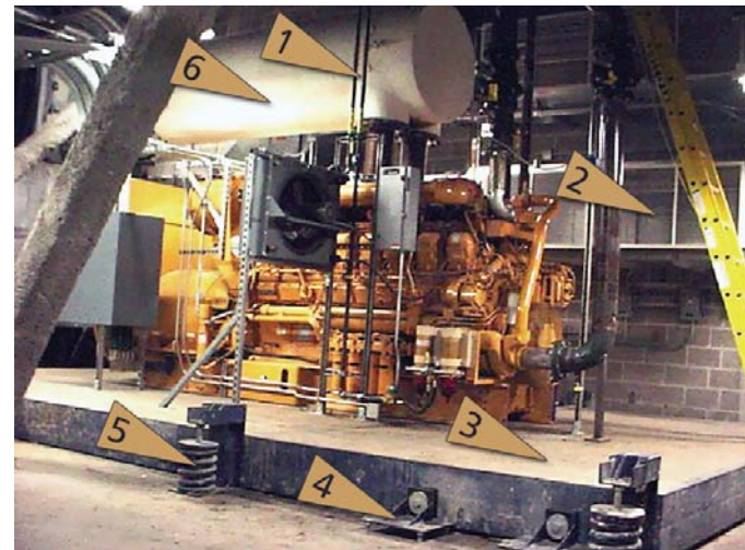
Figure 1: Some key elements of an emergency generator noise and vibration control system:
